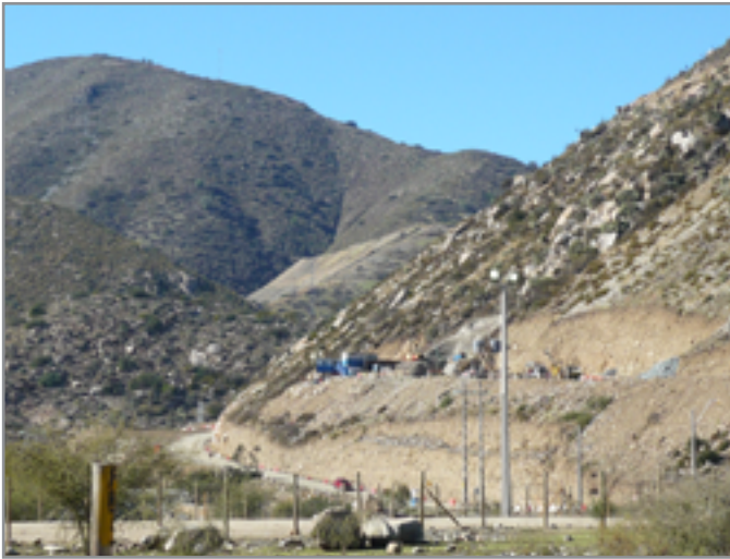
Erosion near a mining road, Pelambres mine, Chile PHOTO: Rocio Avila Fernandez
